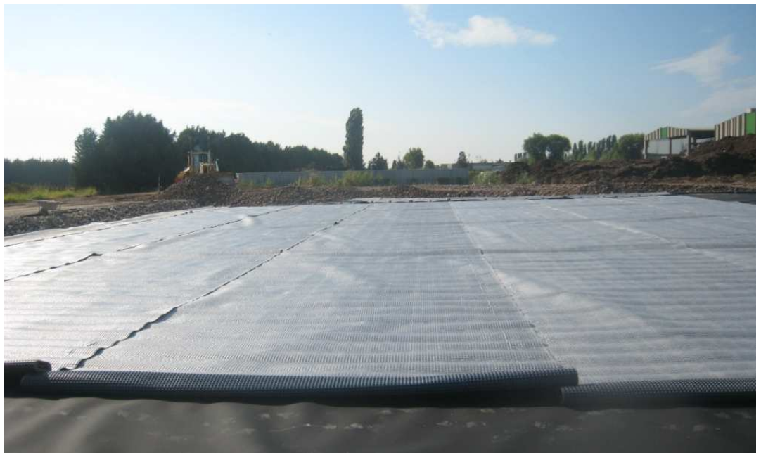
Above geomembrana a studded membrane joined to a nonwoven geotextile is installed, to protect and drain out liquid coming from upper part of closure;
